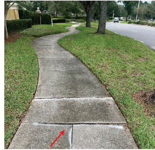
Uneven external sidewalk panels east of unmanned entrance.
