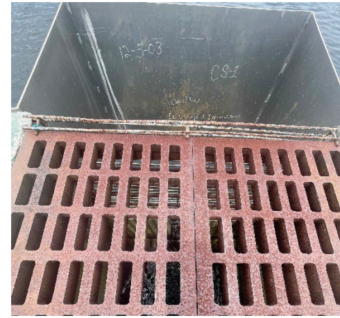
Lake 1 overflow structure with surficial spalling.
