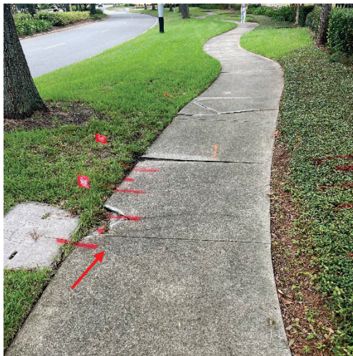
Uneven external sidewalk panels west of unmanned entrance.
