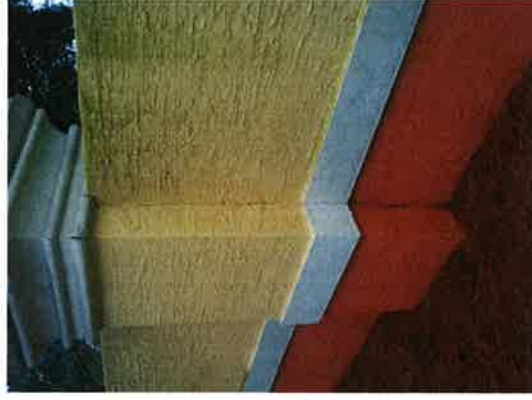
32-Vertical Crack down corner of wall
