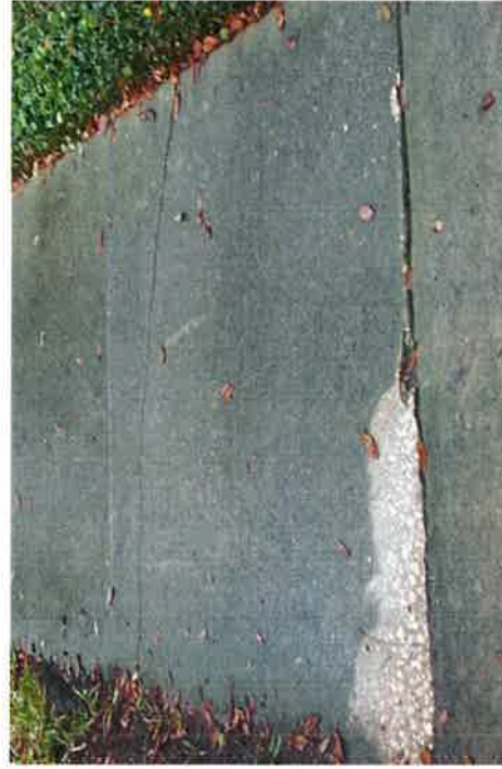
48-Cracking of Sidewalk; grinding down of sidewalk to eliminate deflection
