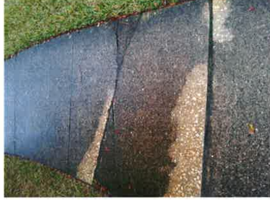
57-Cracking of Sidewalk; grinding down of sidewalk to eliminate deflection
