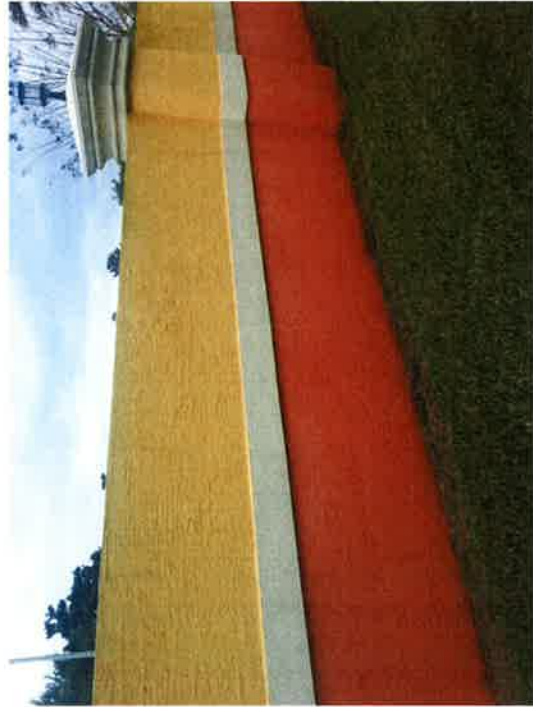
14-Vertical cracks along wall
