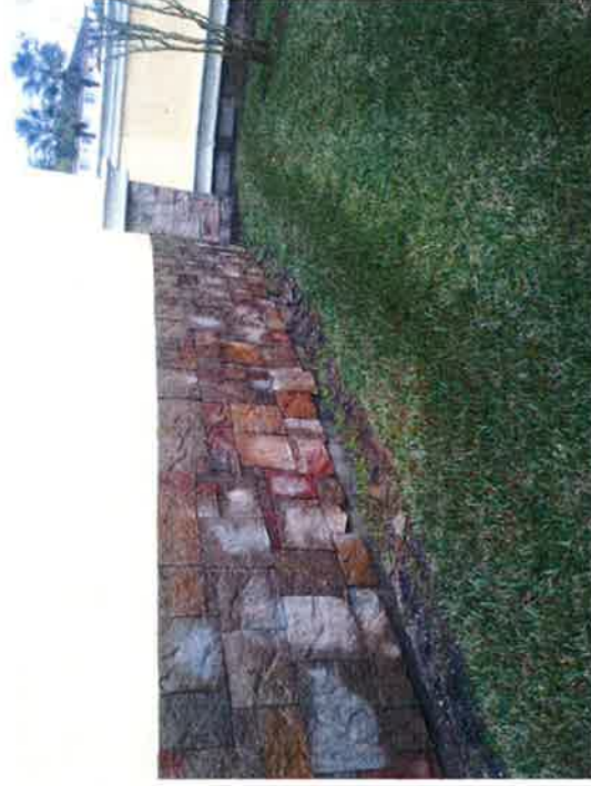
16-Stone facing chipped off or missing from bottom of wall
