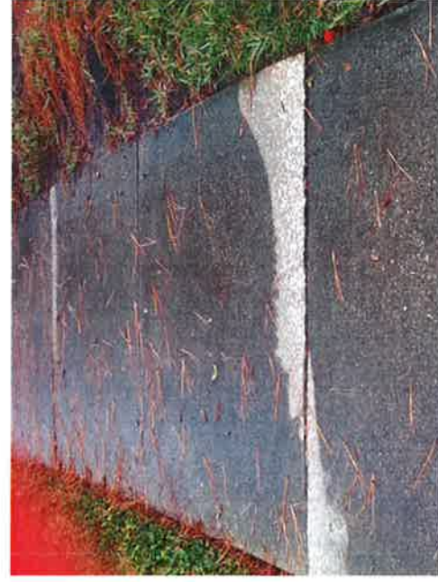
49-Cracking of Sidewalk, grinding down of Sidewalk to eliminate deflection
