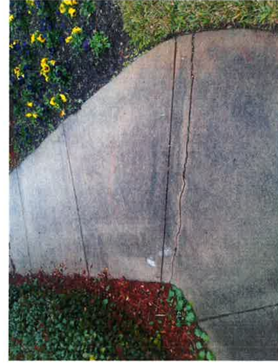
46-Crack in sidewalk
