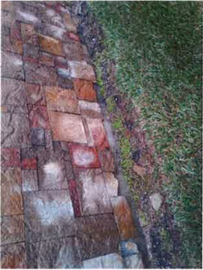
17- Stone facing chipped off or missing from bottom of wall
