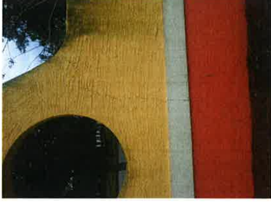
29-Crack down stucco
