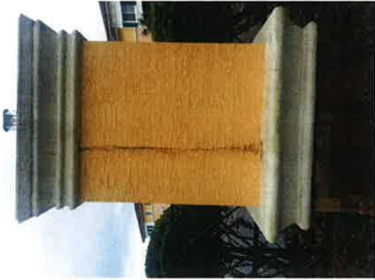
42-Vertical Crack in stucco
