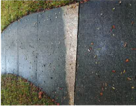
54-Cracking of Sidewalk; grinding down of sidewalk to eliminate deflection
