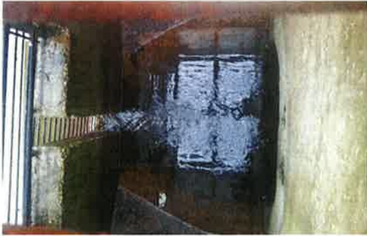
01-Inside of Control Structure for Lake 2
