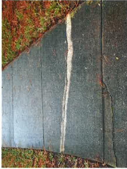
52-Cracking of Sidewalk; grinding down of sidewalk to eliminate deflection
