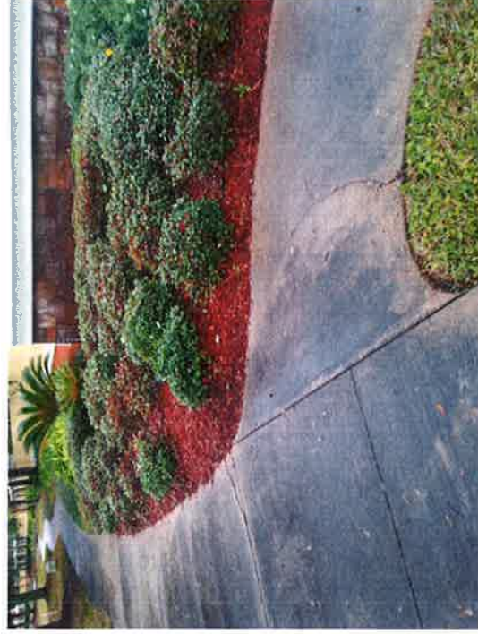
45-Cracking in sidewalk
