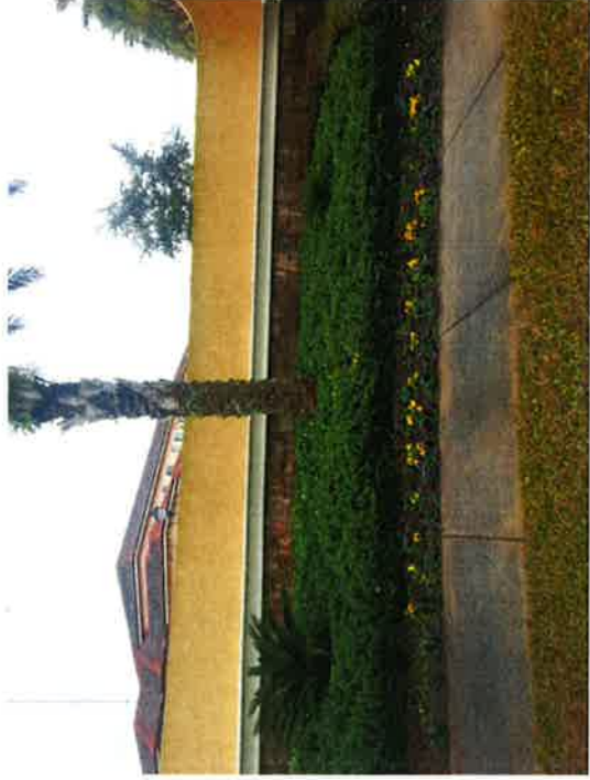
44-Multiple Cracks along stucco of wall
