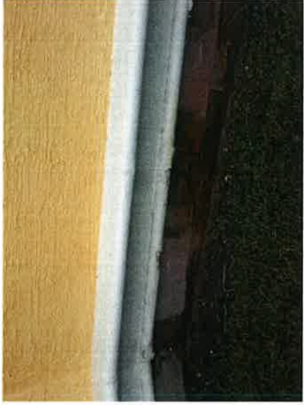
19-Peeling paint and bubbling along stucco
