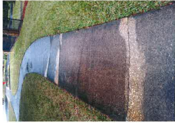
56-Cracking of Sidewalk, grinding down of Sidewalk to eliminate deflection
