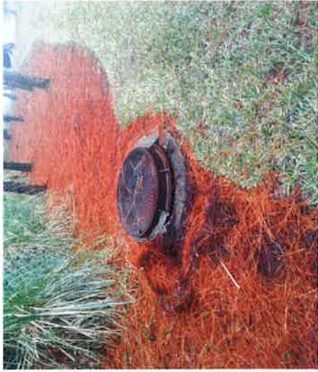
11- Cracked concrete collar around storm manhole
