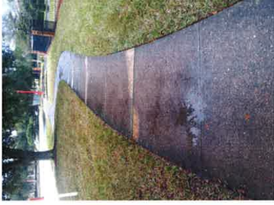
55--Cracking of Sidewalk; grinding down of sidewalk to eliminate deflection
