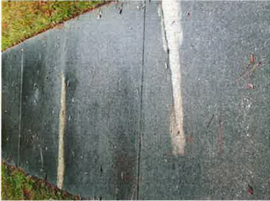
50-Cracking of Sidewalk; grinding down of sidewalk to eliminate deflection
