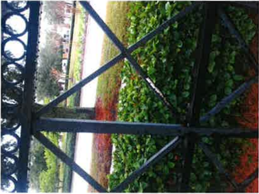
28-Peeling paint on decorative fencing
