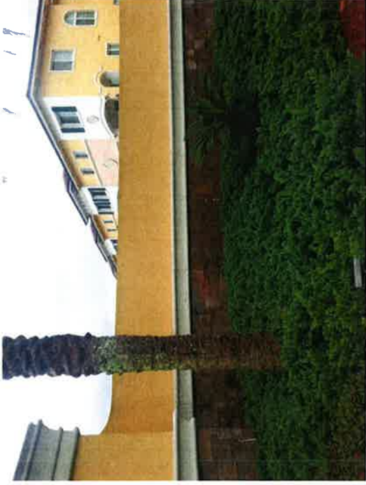
43-Multiple Cracks along stucco of wall
